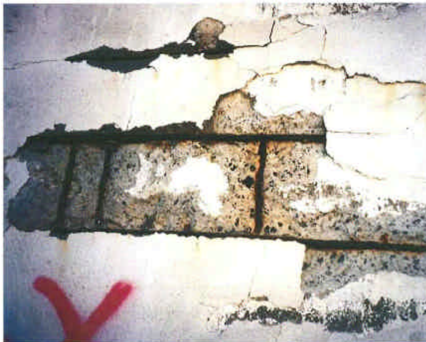
Figure 1 – Area showing severe deterioration, marked for concrete removal.
